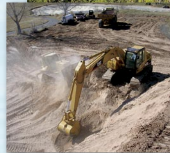
ACI's construction personnel begin work on building a new irrigation lake at Santa Ana Golf Course.
